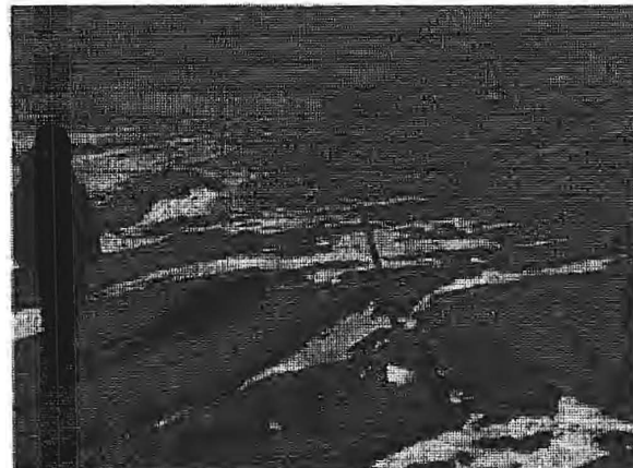
Photo 4 – Downstream slope of the south dam, looking right from the SE corner of the facility. Valve box in the foreground (red arrow) is reportedly for one of two 12” CIP outlet pipelines (other is near the SW corner).
