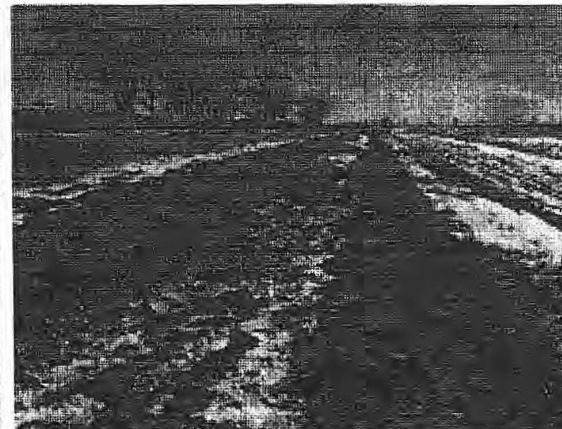
Photo 5 – Downstream slope of the south dam looking left (east). Slope is terraced.
