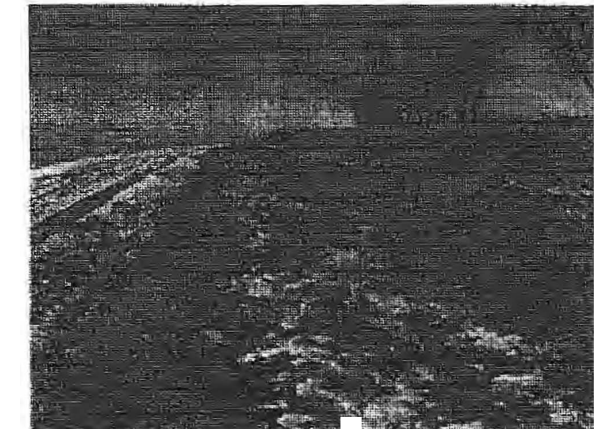
Photo 6 – Downstream slope of south dam looking right near SW corner of the facility.
